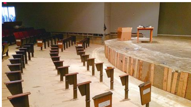
First 3 rows of RCDC auditorium seating after flood
